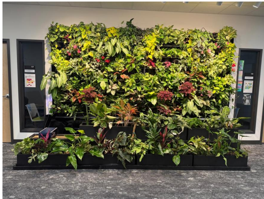
Figure 8. PlantWall in Final Installed Configuration with integrated sensing and irrigation
