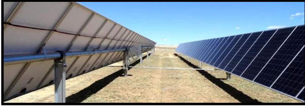
Figure 4: 1p Module Array with Single-Axis Tracking [13]
