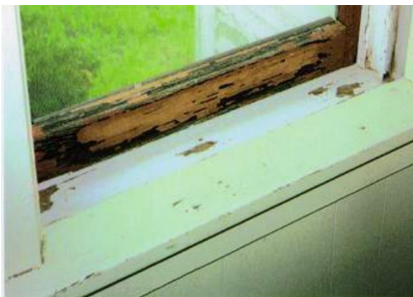
Figure 4.1 —HUD threshold exceeded at window.
