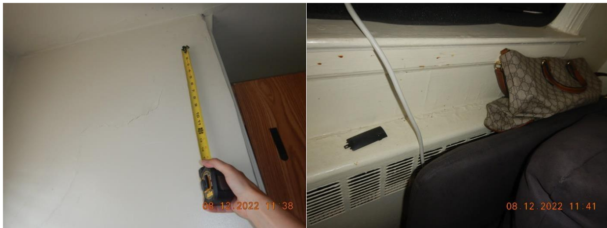
Figures 4.3 and 4.4 (left to right) — Pictures of hazardous levels of paint damage on a wall and heating cover.
