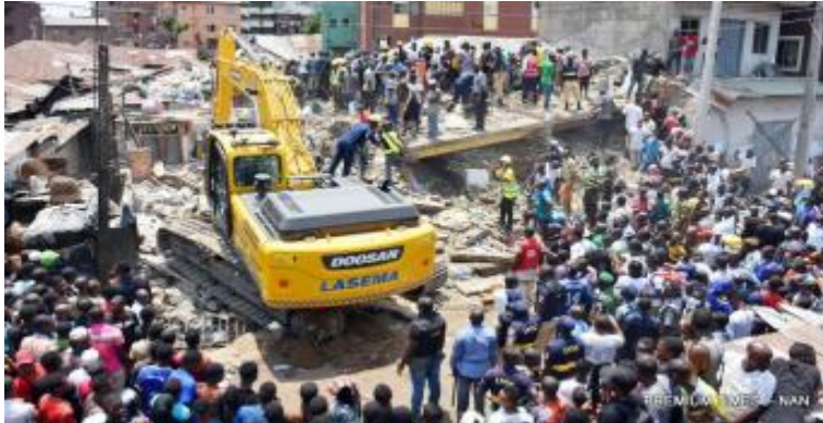
Scene of Ita-faji Building Collapse [16]
