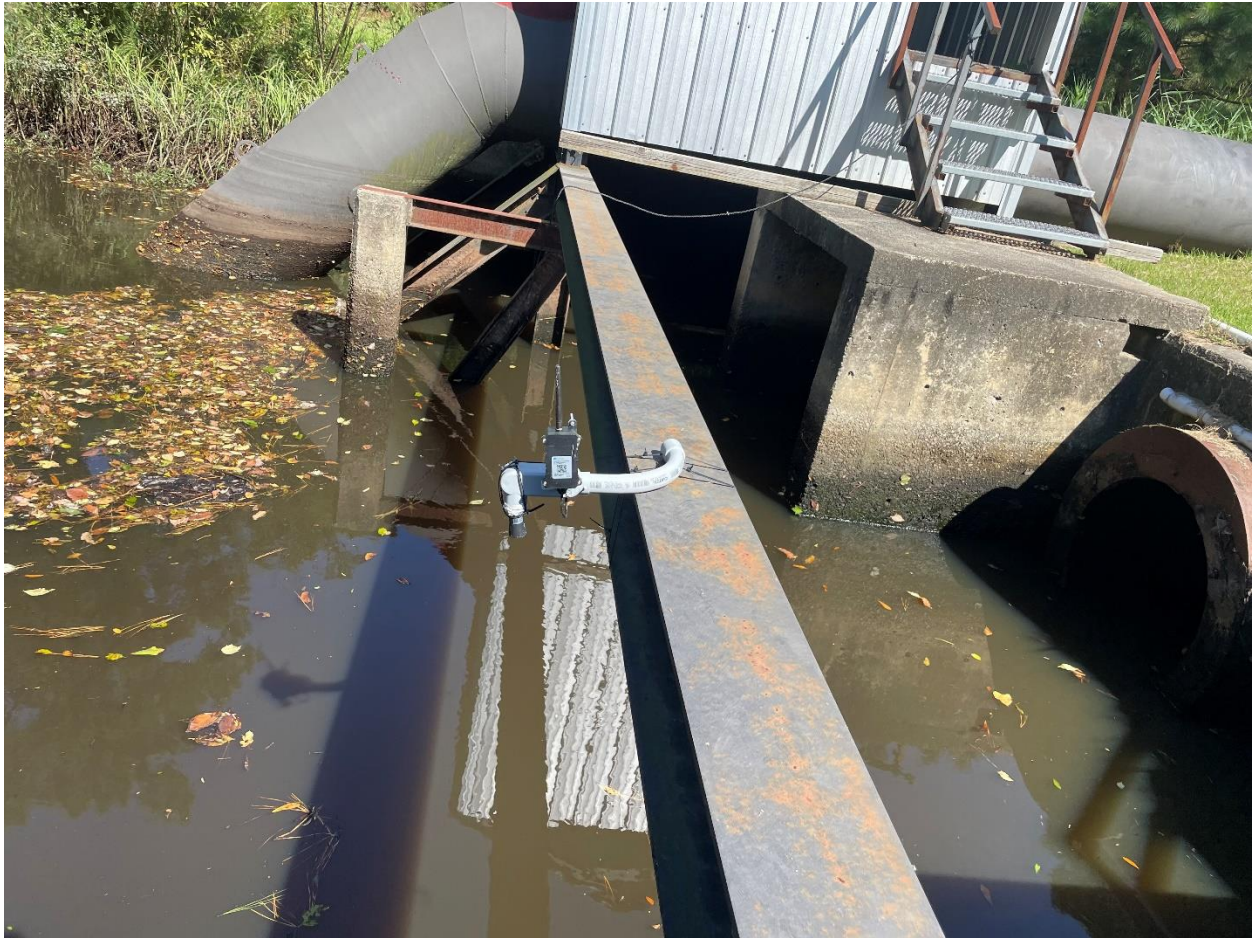
Figure 1, LoRaWAN enabled ultrasound sensor deployed for water level monitoring.
