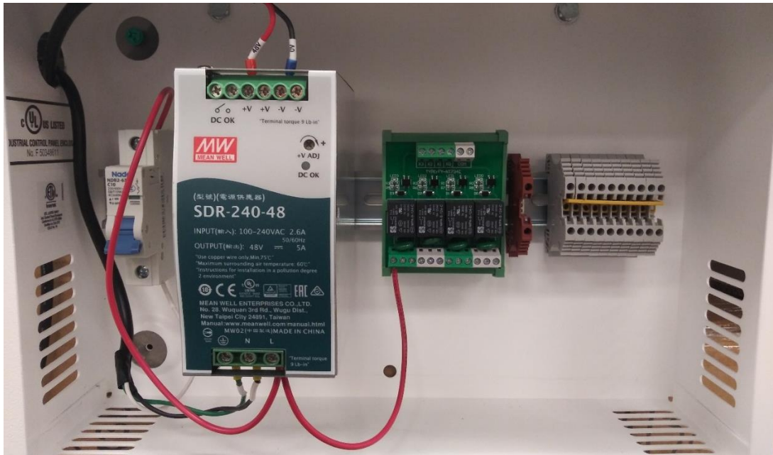
Figure 10. Complete Power Panel Setup
