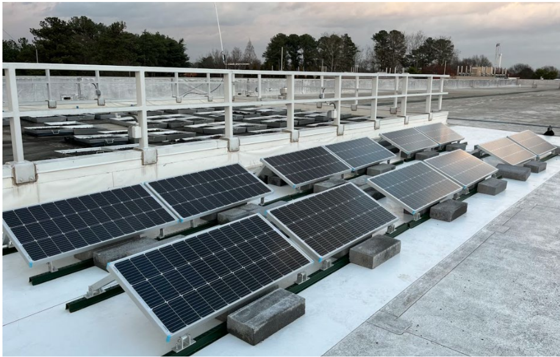
Figure 1. The rooftop PV array with an installed capacity of 1200 Watts.
