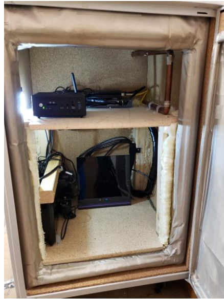
Figure 14: Completed Interior of the Cabinet
