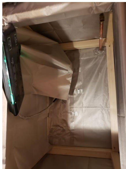
Figure 9: Internal Penetrations in the Cabinet
