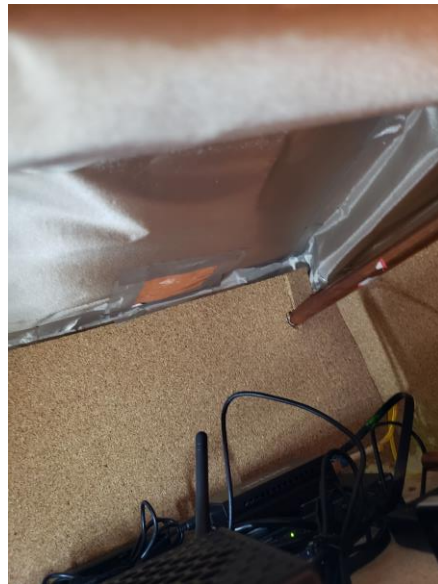
Figure 12: Copper Mesh for the Cabinet's Exhaust
