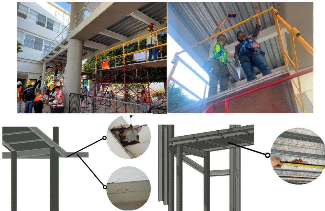
Fig. 10 Visual inspection of localized damage in steel bridge
