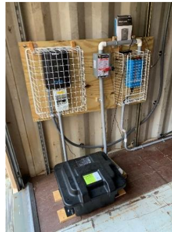
Figure 6: Batteries and Solar Control System
