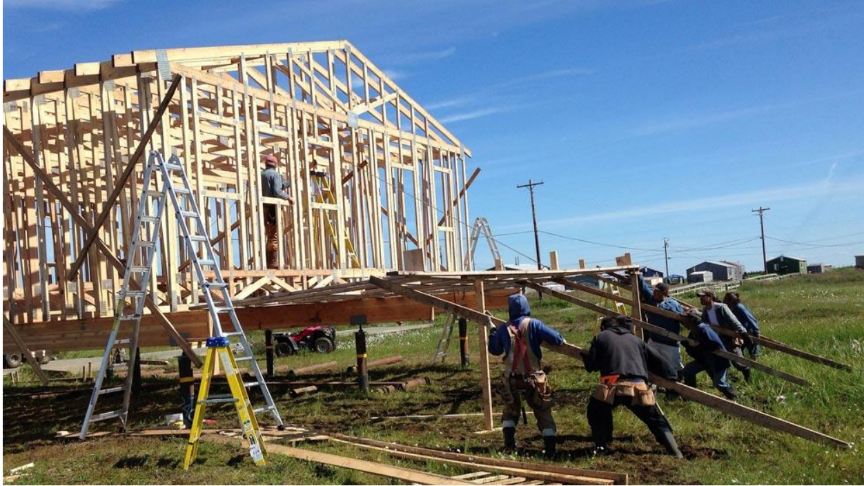
Figure 4. Construction of a home using the integrated truss system. Image courtesy of Cold Climate Housing Research Center, Inc.
