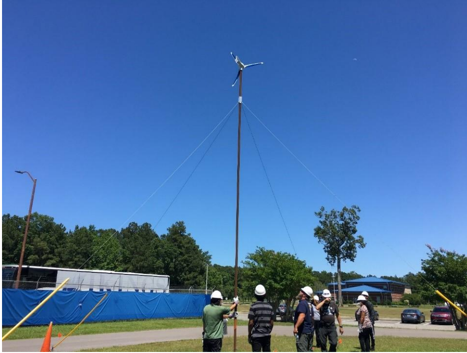
Photo 5. A fully installed wind turbine
